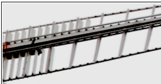
Missing shutters still to be fitted
